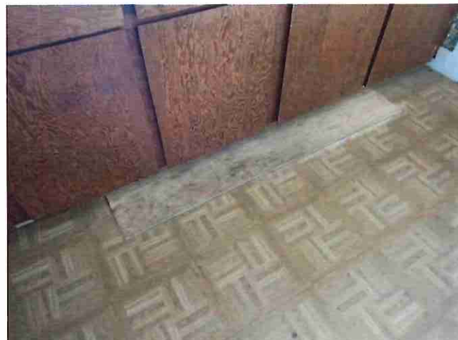
Missing Floor Covering
