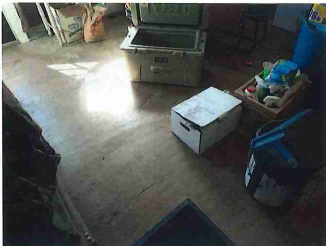
Missing Floor Covering
