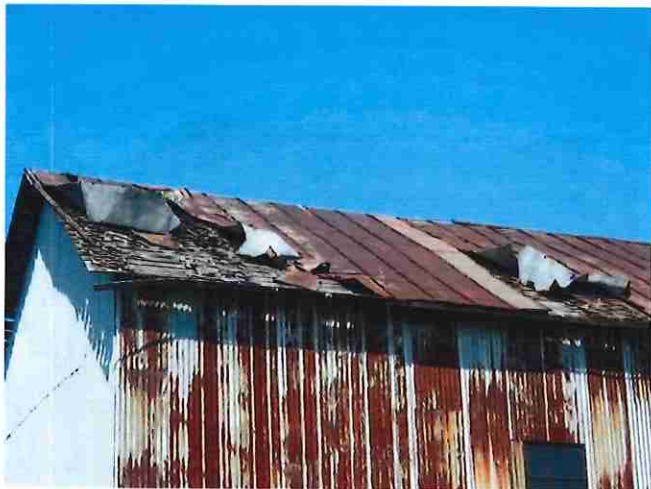
Dilapidated Barn Roof
