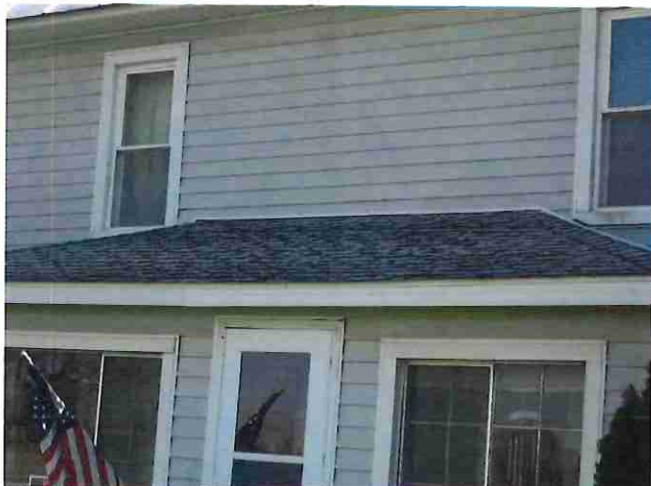
Worn Roof Shingles
