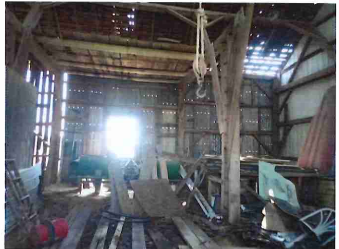
Dilapidated Barn Interior
