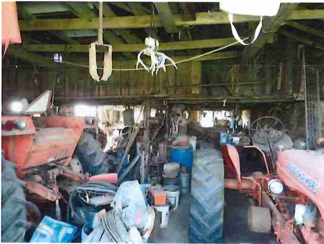
Dilapidated Barn Interior
